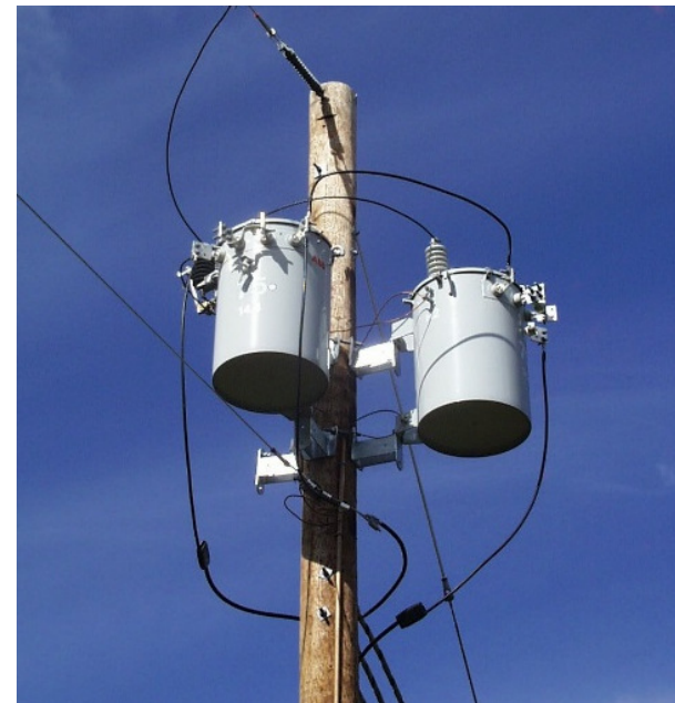
480 Volt, 1Ø utility service may be provided using two(2) conventional 240 Volt, 1Ø Transformers
